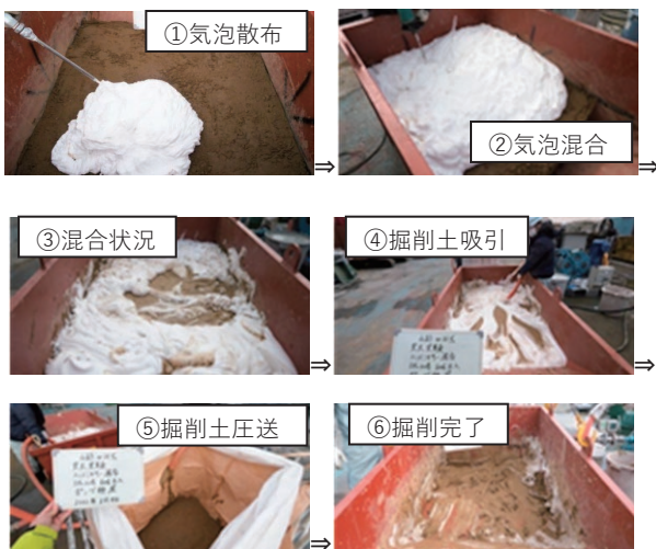
Photo 4 気泡を用いた掘削作業の省力化 (Effortless Excavation Procedure with Fine Bubble Mixing)
