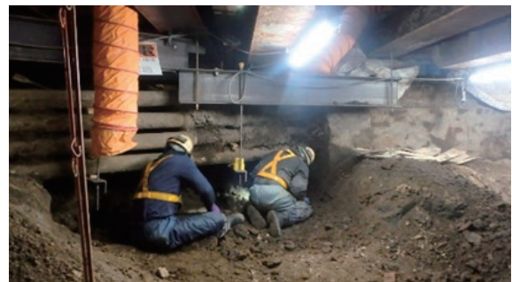
Photo 1 ライフライン直下での掘削作業 (The Workers Struggled in Excavation Beneath the Lifelines)
