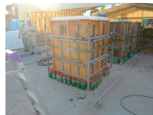
Photo 4 模擬部材試験体製作状況 (Production Status Compressive Strength Specimen for Simulated Members)
