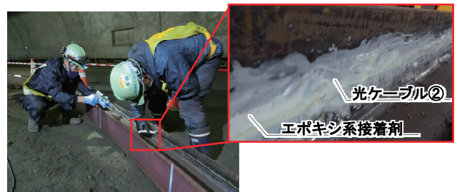
Photo 1 鋼製支保工への貼付け (Optical Fiber Cable Placed on Steel Support)
