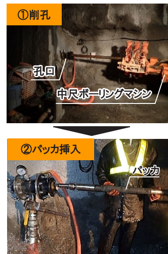
Photo 3 中尺スイリモ適用状況 (新北陸トンネル) (Moderate-Length Boring and Measurement of water pressure at Shin-Hokuriku Tunnel)
