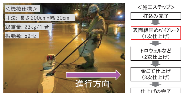
Photo 1 表面締固めバイブレータの仕様及び施工手順 (Specifications and Construction Process of Surface Compaction Vibrator)
